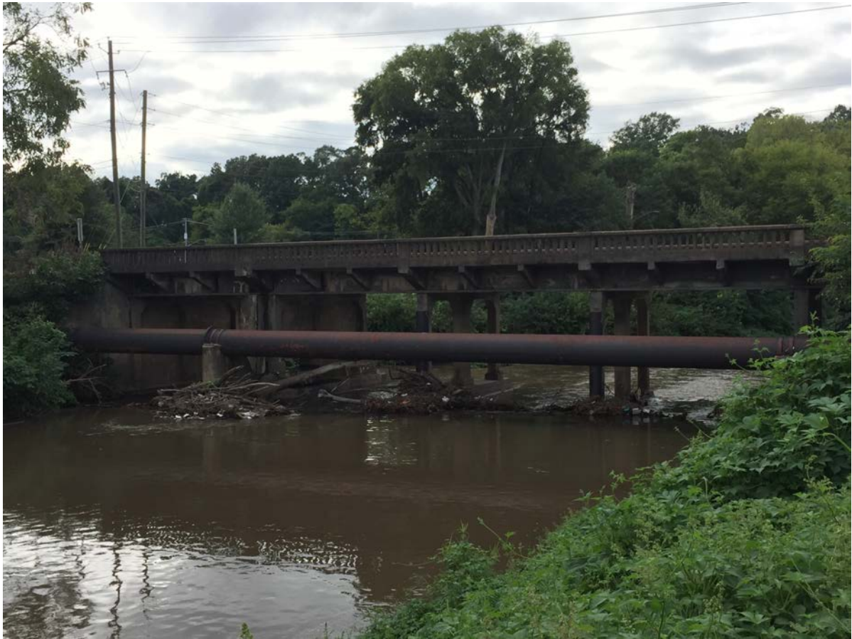
Image 1-1: Avenue F Bridge at Village Creek. Note accumulated debris at sewer line support structure.
