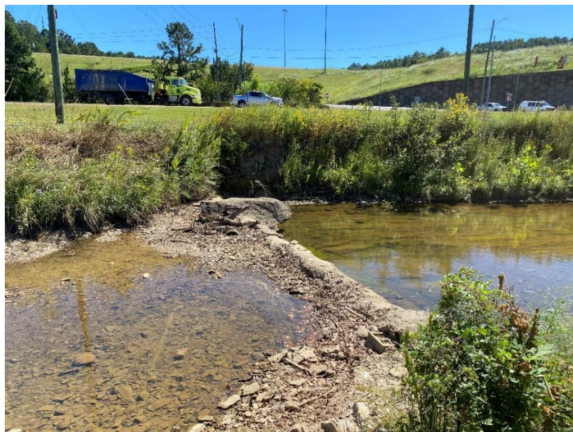
Photo 3: View of Sanitary Sewer Line crossing Shades Creek, just north of Crestwood Boulevard
