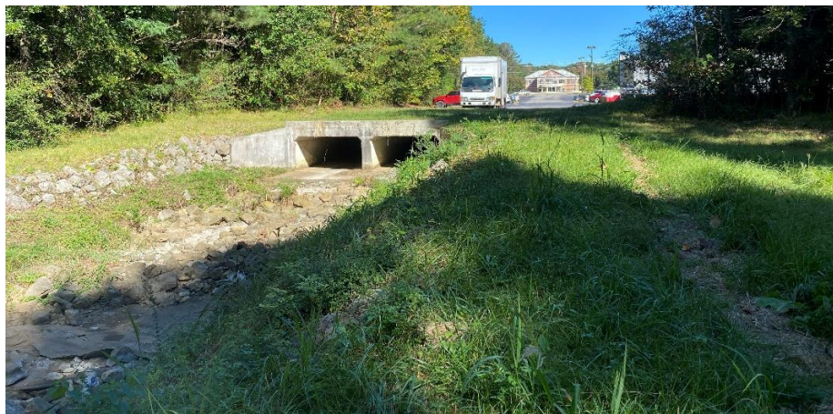
Photo 18: Headwall and Drainage Channel at Southwest Corner of Winn Dixie Parking Lot
