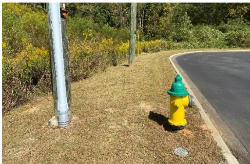
Photo 21: Utilities along Northwestern Edge of Hobby Lobby Parking Lot
